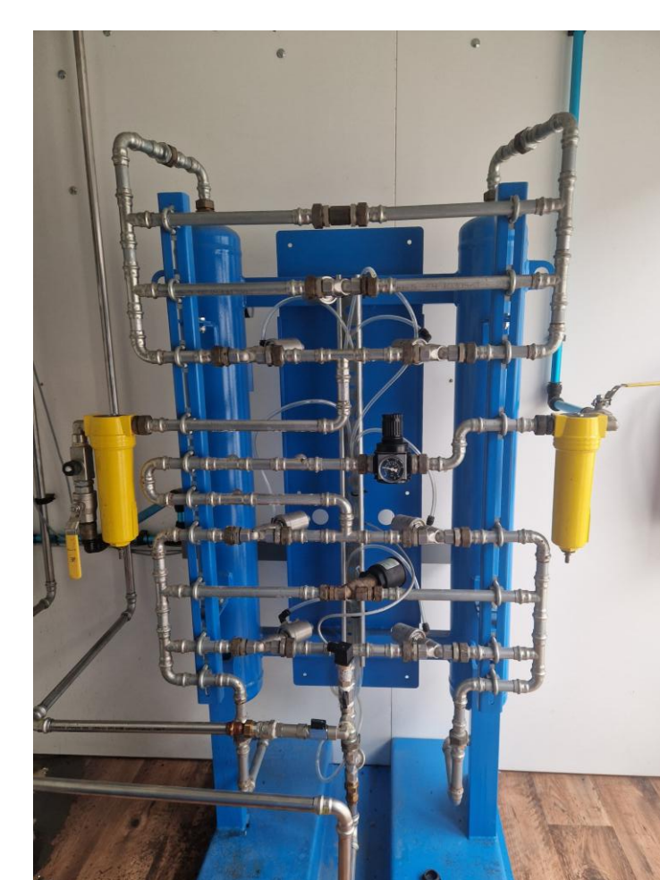
Figure 2. Pressure Swing Adsorption (PSA) system for upgrading biogas to biomethane.
