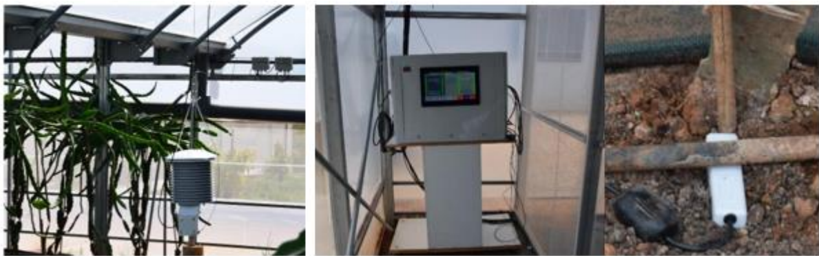
Figure 8: Inderen ATMOS-14, TEROS-11 and Control Cabinet.
