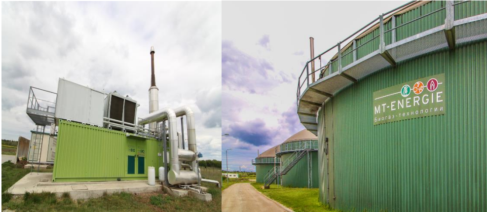
Figure 14. Close-up view of a part of the biogas facility.
